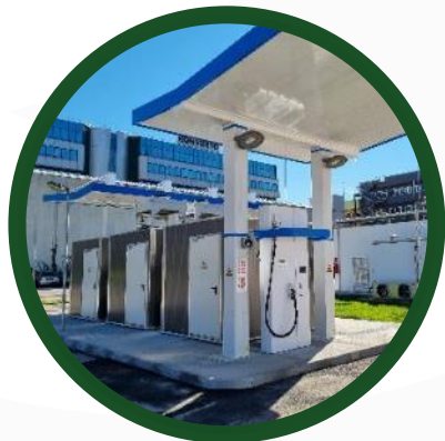
Hydrogen Smart Container & Refueling Station
