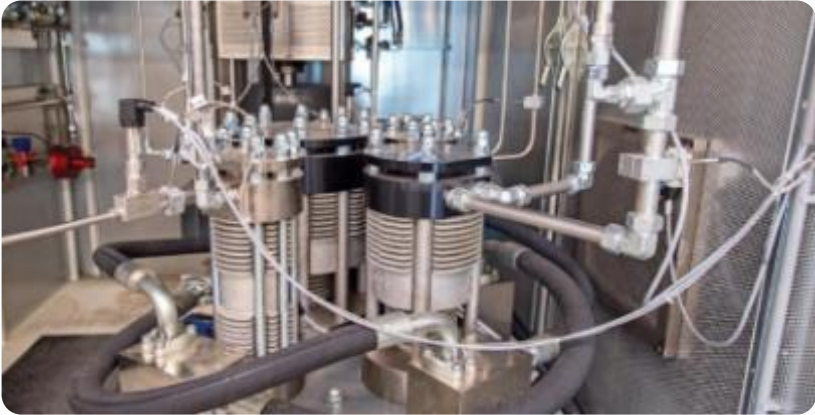
| Hydrogen production plant
